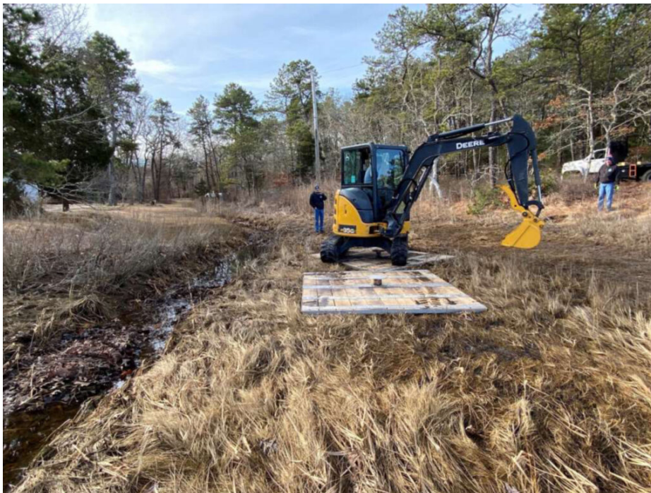
Plymouth County Mosquito Control Project excavator. Photo courtesy of Plymouth County Mosquito Control Project.
